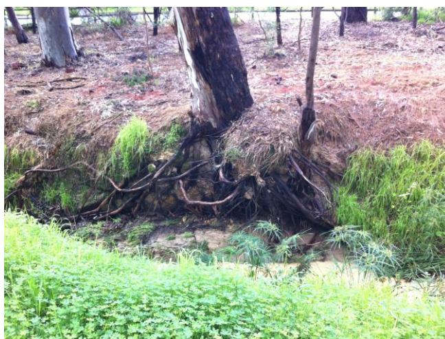
Exposed roots of a mature SA Blue Gum located on the creekline in the vicinity of the proposed Site 11 works. This tree is in danger of being lost due to erosion.
